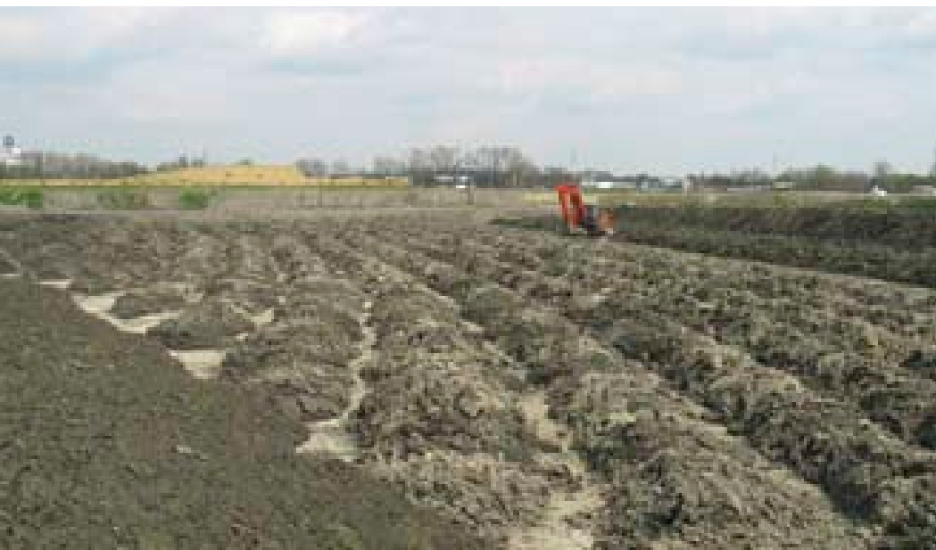
Figure 2. Dredged material being dried and worked upon at the Fasiver site. A total of 1.3 million tdm will be processed.
