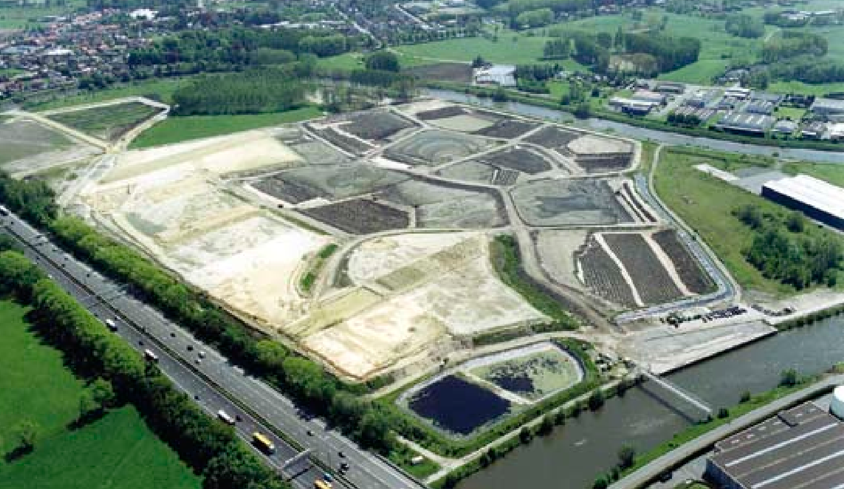
Figure 1. Aerial view of the Fasiver site in the process of being treated with millions of tonnes of clean dredged material.
