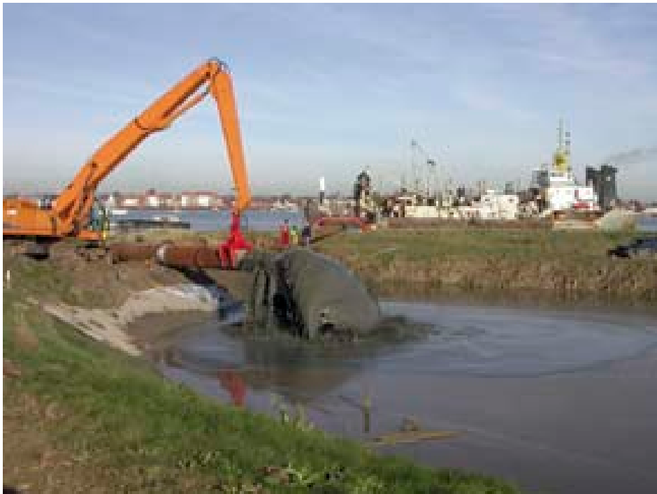
Figure 4. The dredged material was pumped through a pipeline from the vessel into a containment bund on the seaward side of the new seawall.
