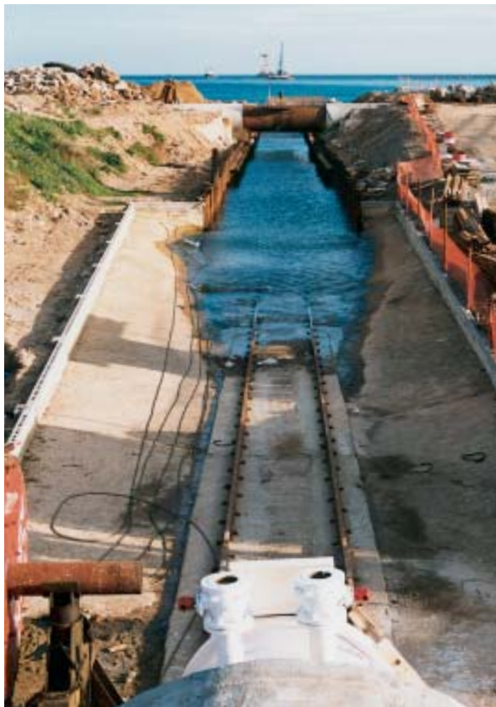
Figure 11. In the foreground, the pipeline is awaiting the pull. In the background is the pull barge and the pontoon dredging underneath the gas line. In the middle ground is a sewer diversion pipe crossing the pipe trench.
