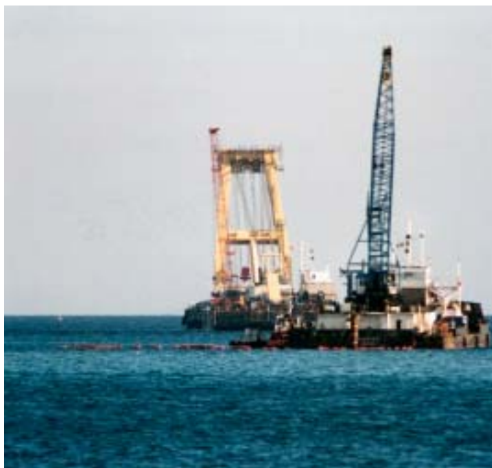
Figure 4. After backfilling, the area was compacted using twin torpedo vibro-compactors supported from the crane barge Kutxa . Kutxa is seen here dredging under the gas line, with a pull barge behind.
