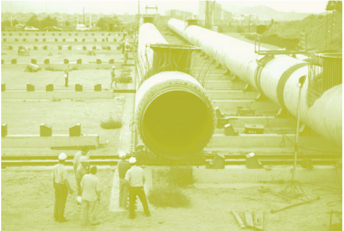
Figure 2. The first pipe string being moved from the welding area to the stock area. The structures on top of the pipe are the starters for the diffusers.
