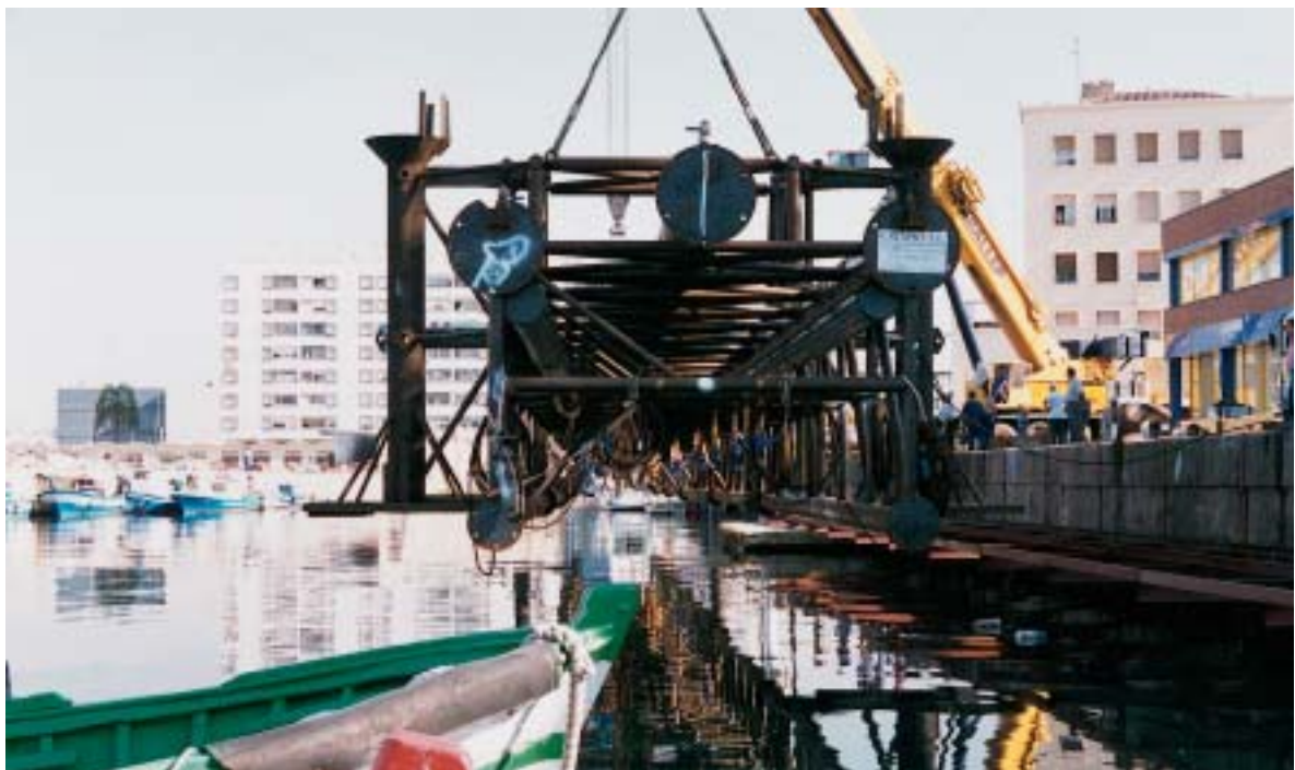
Figure 6. The gas pipeline bridge is lowered into the harbour in preparation for towing out to site. This support bridge is 60 m overall length.
